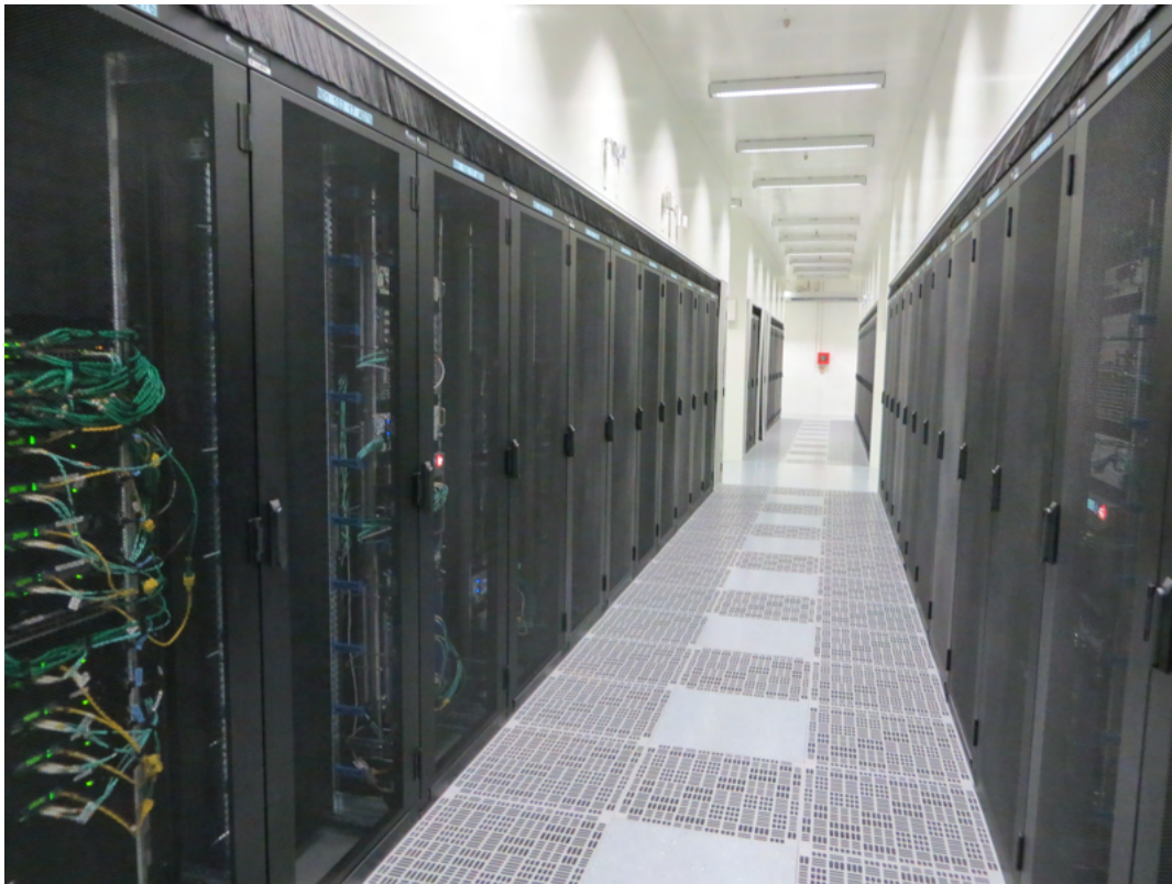
FIGURE 1.1 – DCs servers room with cold air distributed through the raised floor. The picture was taken in Orange’s DC in Val De Reuil, in 2013.
